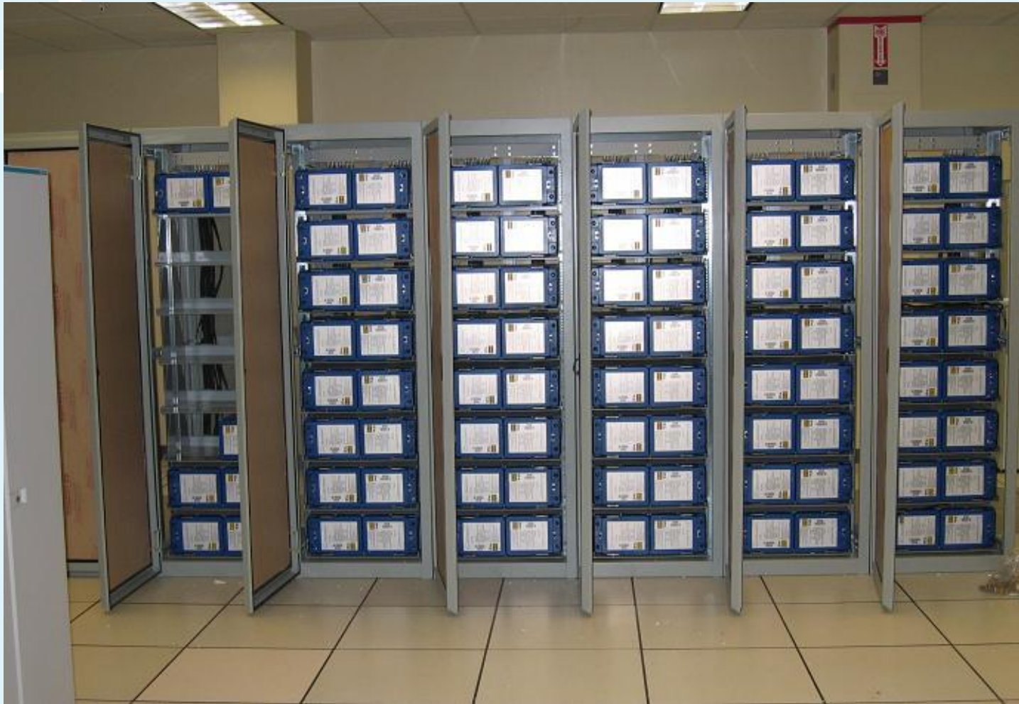
Data Center Installation
