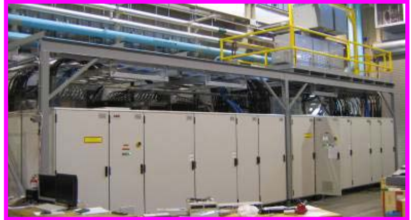
6.25 MVA / 5 MW Variable Voltage Source (VVS) Converter “Amplifier”
