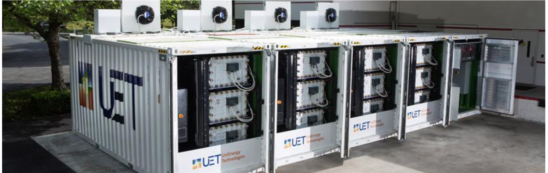
1 MW installation in Pullman, WA for Avista
