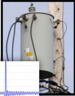
Failing Pole Top Transformer
