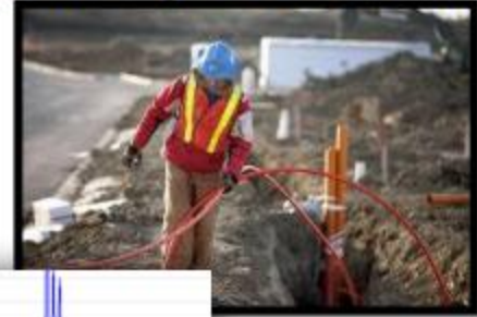
Failing Underground Cable
