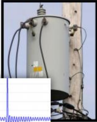
Failing Pole Top Transformer
