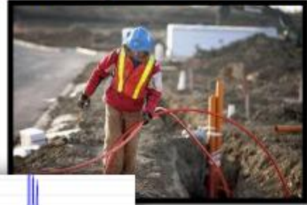
Failing Underground Cable
