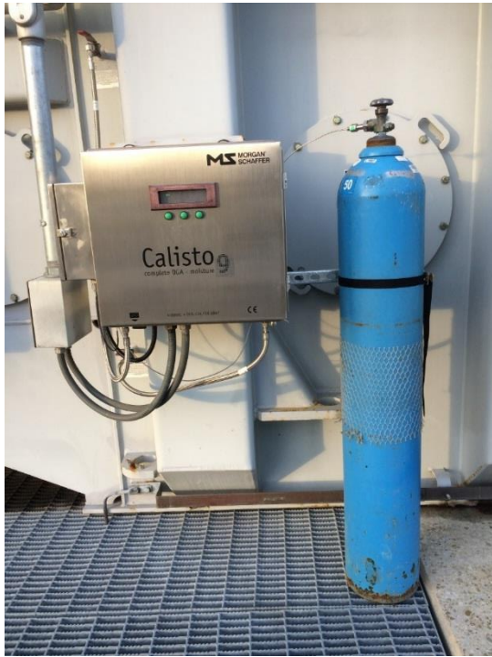
7 Gas Dissolved Gas Analysis Monitoring Unit
