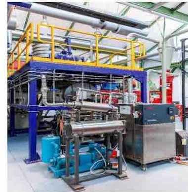
Figure 7 – Black Mass (Powder) Vacuum Dryer, Condenser and Electrolyte Recovery Circuit
