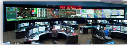
Power Control Center
