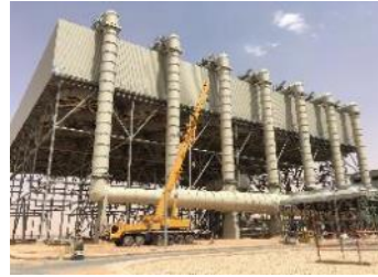
Air Cooler Condenser Unit
