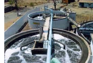
Effluent Treatment Plant
