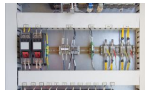
Control Systems Integration
