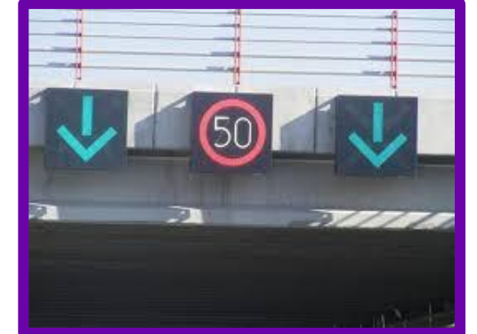
2220+ Lane Control Signs (LCS)
